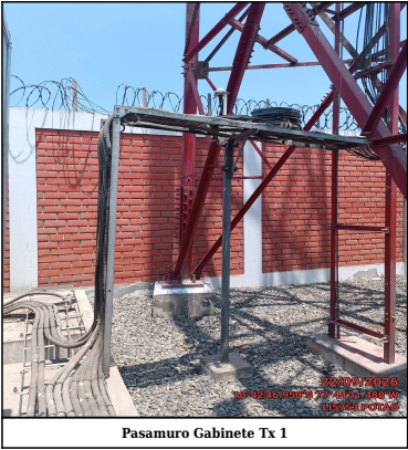
Pasamuro Gabinete Tx 1
