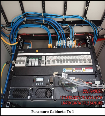
Pasamuro Gabinete Tx 1
