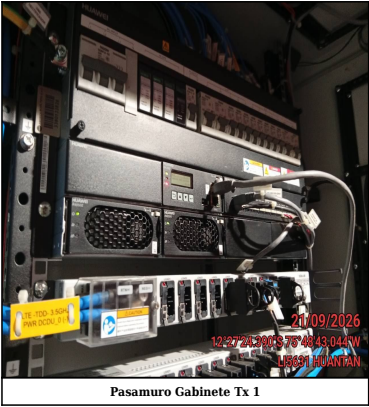
Pasamuro Gabinete Tx 1
