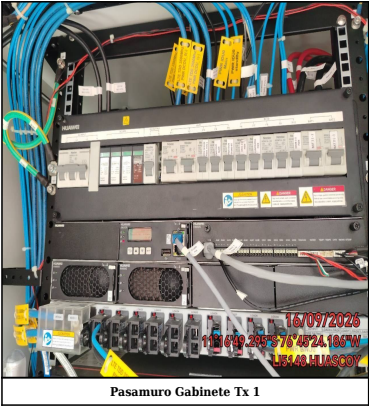
Pasamuro Gabinete Tx 1
