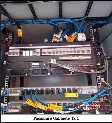
Pasamuro Gabinete Tx 1
