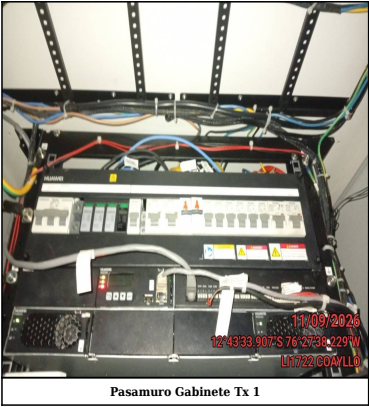
Pasamuro Gabinete Tx 1
