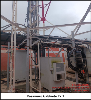
Pasamuro Gabinete Tx 1
