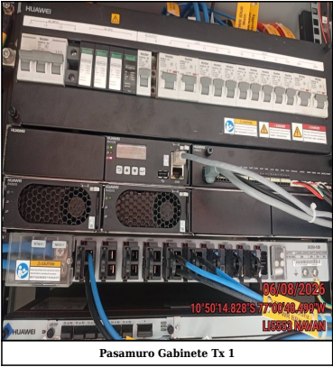
Pasamuro Gabinete Tx 1
