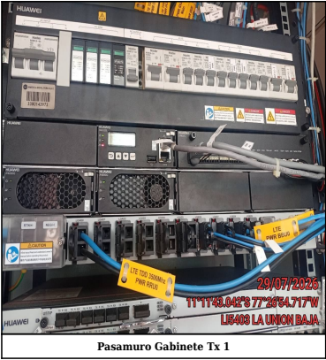
Pasamuro Gabinete Tx 1
