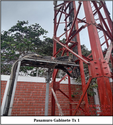
Pasamuro Gabinete Tx 1
