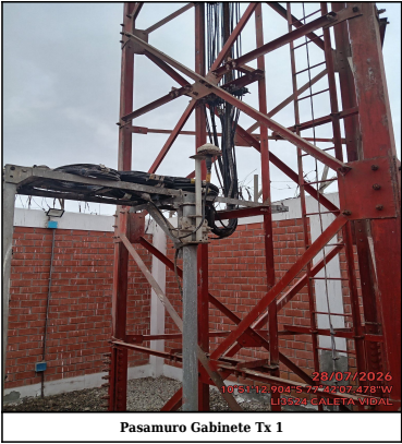
Pasamuro Gabinete Tx 1
