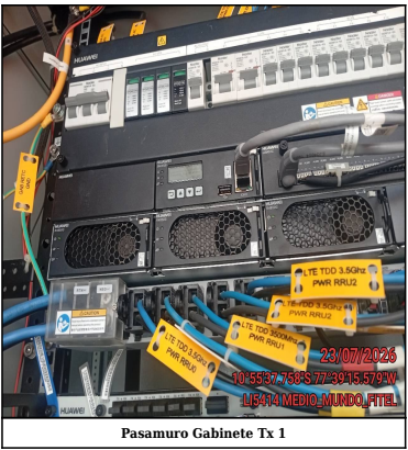
Pasamuro Gabinete Tx 1
