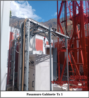
Pasamuro Gabinete Tx 1
