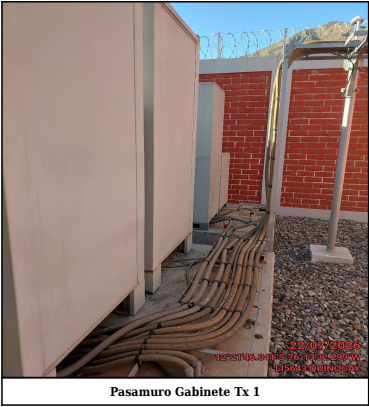
Pasamuro Gabinete Tx 1
