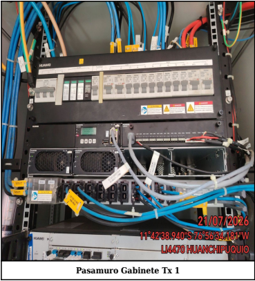
Pasamuro Gabinete Tx 1
