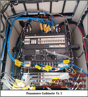
Pasamuro Gabinete Tx 1
