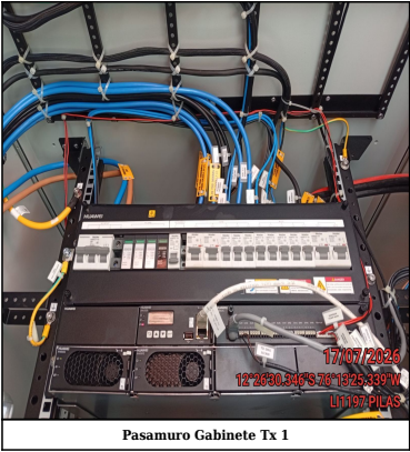
Pasamuro Gabinete Tx 1
