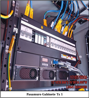
Pasamuro Gabinete Tx 1
