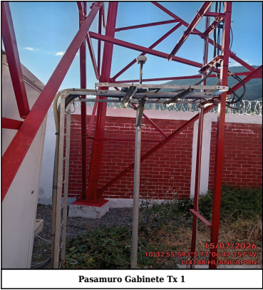
Pasamuro Gabinete Tx 1
