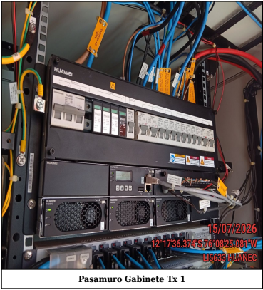
Pasamuro Gabinete Tx 1
