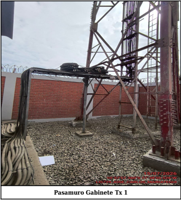
Pasamuro Gabinete Tx 1
