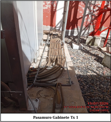
Pasamuro Gabinete Tx 1
