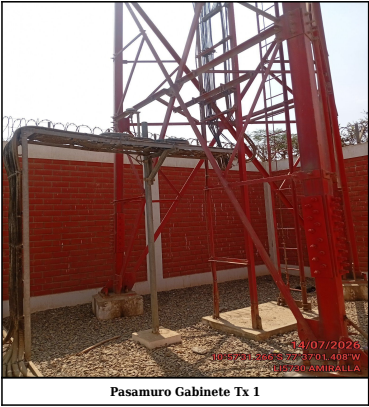
Pasamuro Gabinete Tx 1
