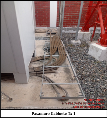
Pasamuro Gabinete Tx 1
