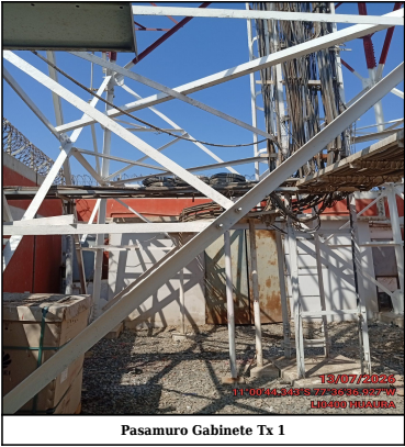
Pasamuro Gabinete Tx 1
