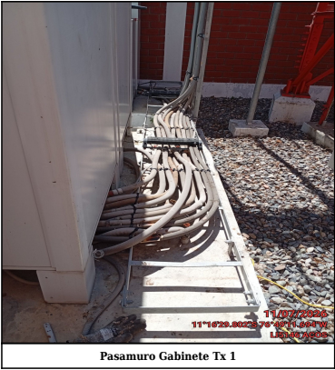
Pasamuro Gabinete Tx 1
