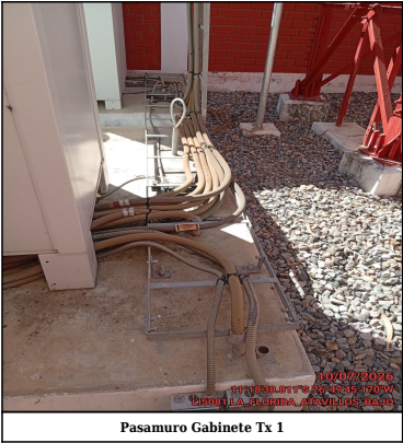
Pasamuro Gabinete Tx 1
