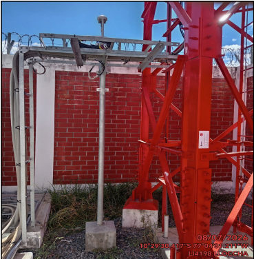
Pasamuro Gabinete Tx 1
