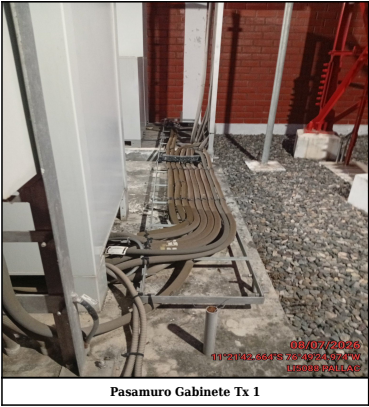
Pasamuro Gabinete Tx 1
