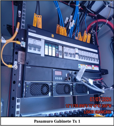
Pasamuro Gabinete Tx 1
