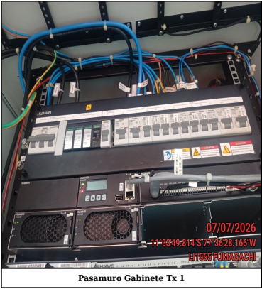
Pasamuro Gabinete Tx 1
