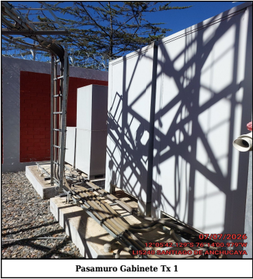
Pasamuro Gabinete Tx 1
