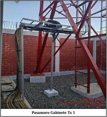
Pasamuro Gabinete Tx 1
