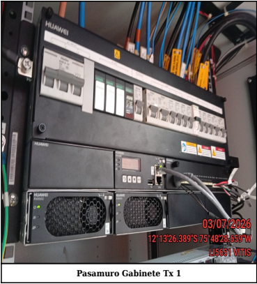
Pasamuro Gabinete Tx 1
