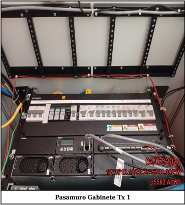
Pasamuro Gabinete Tx 1
