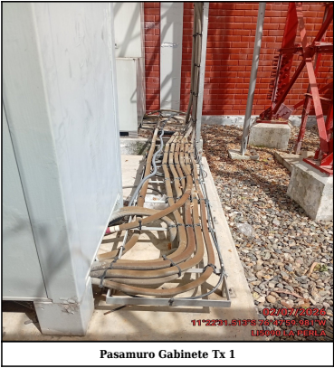
Pasamuro Gabinete Tx 1
