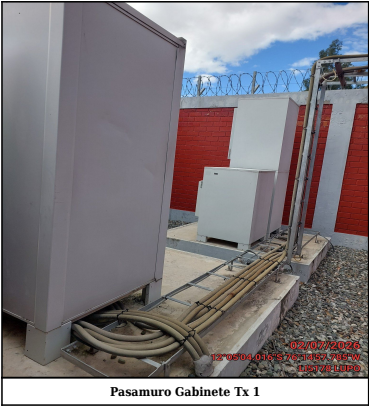
Pasamuro Gabinete Tx 1
