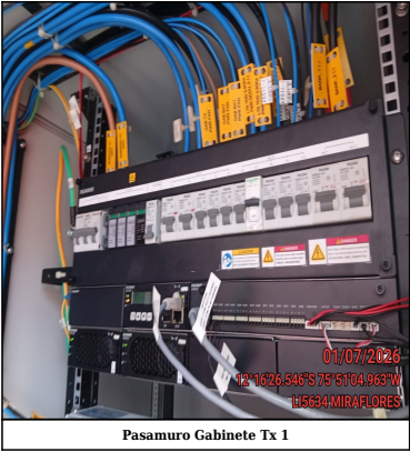
Pasamuro Gabinete Tx 1
