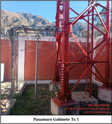
Pasamuro Gabinete Tx 1
