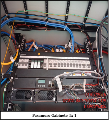
Pasamuro Gabinete Tx 1
