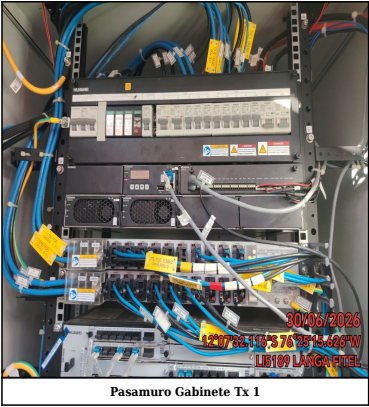
Pasamuro Gabinete Tx 1
