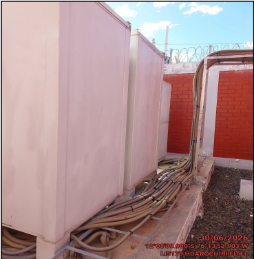
Pasamuro Gabinete Tx 1
