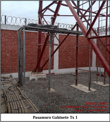
Pasamuro Gabinete Tx 1
