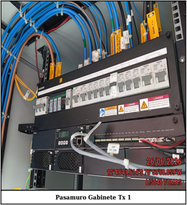
Pasamuro Gabinete Tx 1
