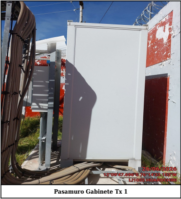
Pasamuro Gabinete Tx 1
