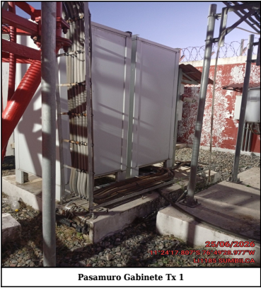
Pasamuro Gabinete Tx 1
