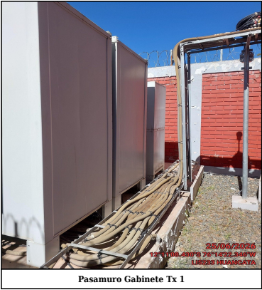
Pasamuro Gabinete Tx 1
