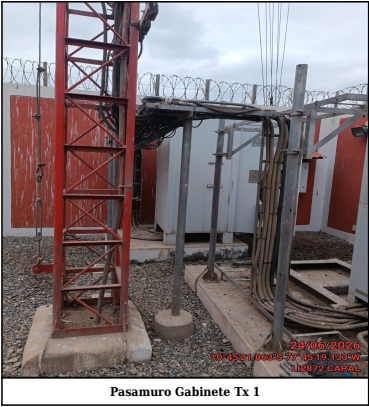
Pasamuro Gabinete Tx 1
