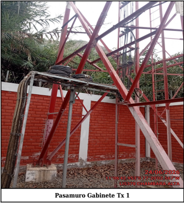
Pasamuro Gabinete Tx 1
