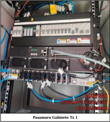
Pasamuro Gabinete Tx 1
